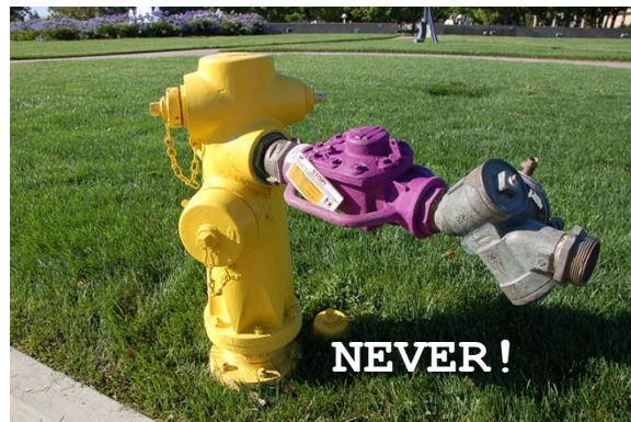
Figure 5: Incorrect RW hydrant and meter hook-up
