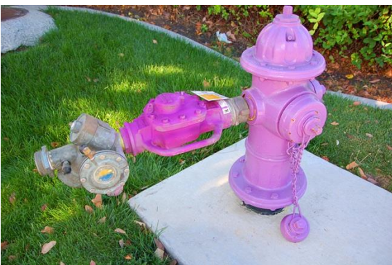
Figure 4: Correct RW hydrant and meter hook-up
