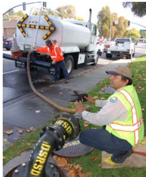
Water Operators Ray Robles (front) and Bill Smith (rear) prepare to test an emergency connection to EBMUD's water system by flushing sediment from the rarely used pipes.
