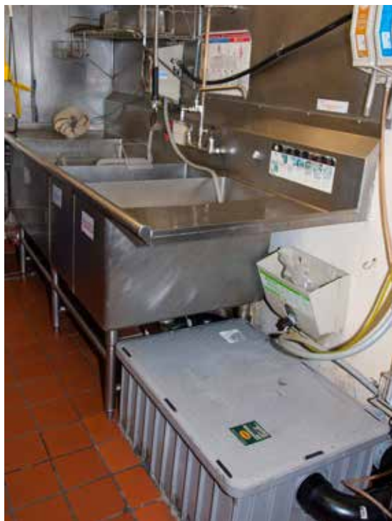
The gray box on the floor is a grease trap located inside a commercial kitchen.
