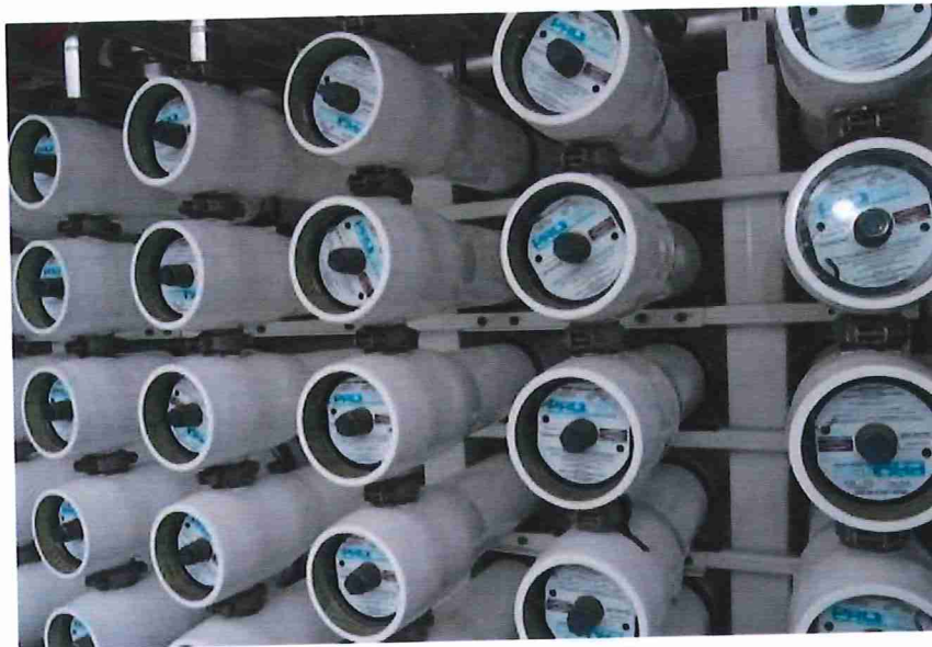
Bank of Desalination Membrane Filtering Tubes
