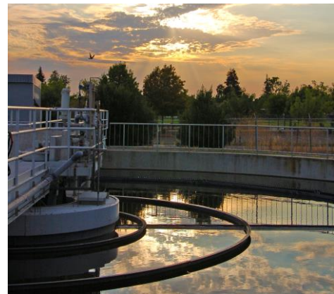
DSRSD uses four secondary clarifiers to remove "spent" microorganisms from treated wastewater effluent.
