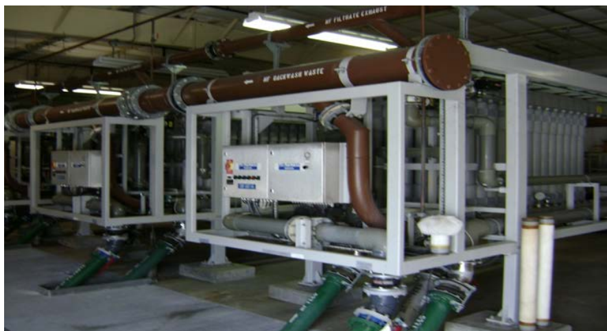
Five microfiltration units remove all particles greater than 0.2 microns.
