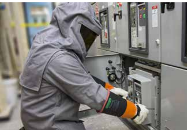
Electrician II Brian Johnson installs a power distribution circuit breaker into an energized 480V distribution switchgear.
