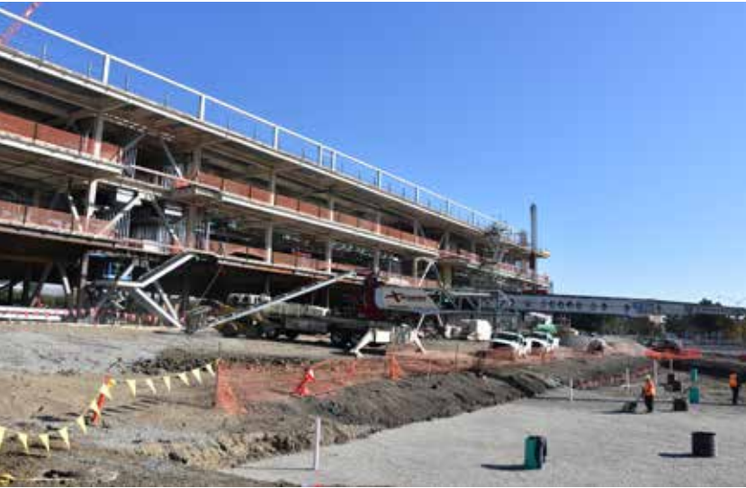
Construction is underway at Carl Zeiss' U.S. headquarters on Dublin Blvd. The 13.5-acre site will house Zeiss Medical Technology group, the company's Industrial Quality & Research branch, and its Semiconductor Manufacturing Technology division.
