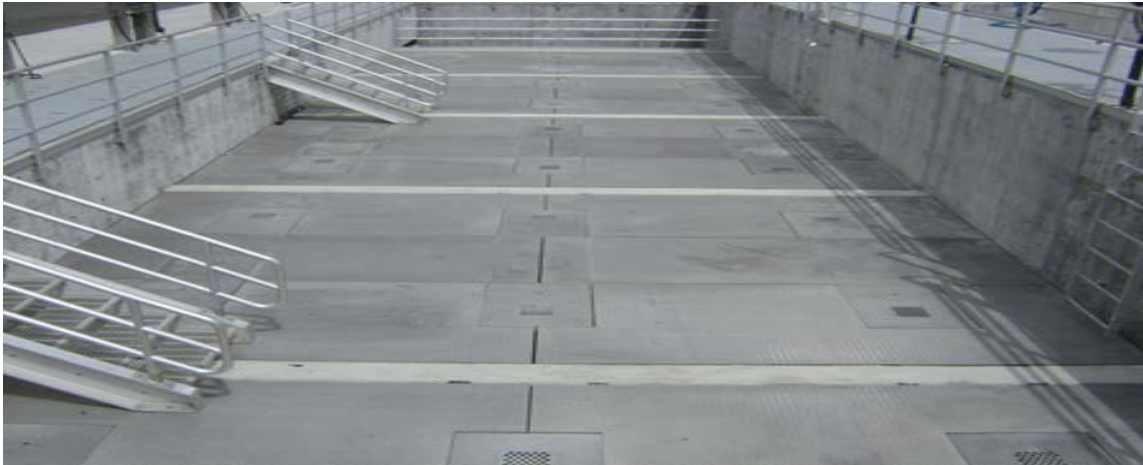
Access plates hide six sand filters where flocculated water flows upward through 80 inches of continuously backwashed sand.
