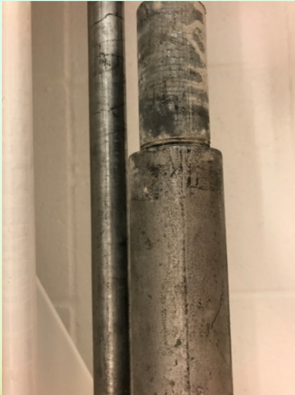
The exterior of the conduit pipe appears to be in good condition
