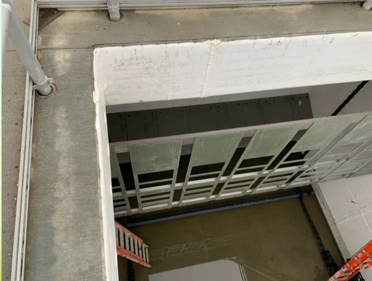
Photo taken of baffles recently installed at the Sunnyvale Wastewater Treatment facility
