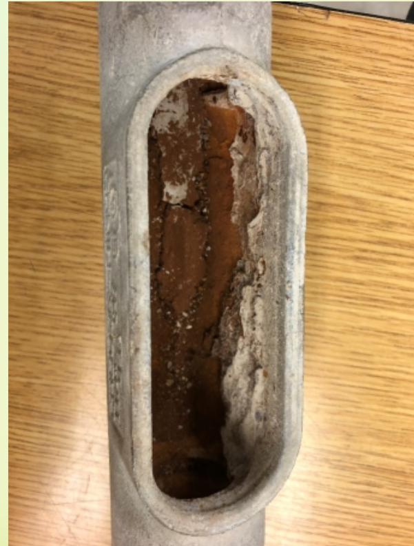
The interior of the conduit pipe shows it is corroding from the inside - out
