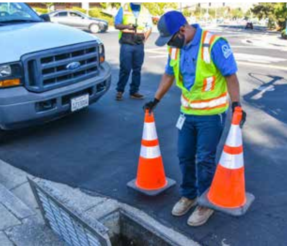
DSRSD staff has continued to work throughout the pandemic. Water/Wastewater Operator Systems III Alex Ortega is wearing a face covering while he works at the site of a pipe leak.
