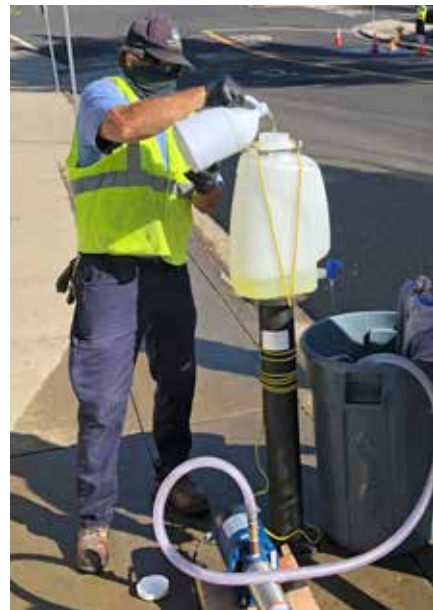
Water/Wastewater Systems Operator II Tim Johnson adds chlorine to disinfect a new portion of 8-inch water main on Southwick Drive in Dublin in October 2020.
