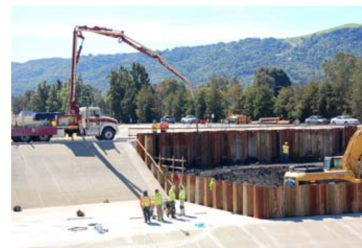
Contractors pour cement April 18 to create an enclosure for new pretreatment equipment at the Jeffrey G. Hansen Water Recycling Plant in Pleasanton, part of an $18.2 million project that will boost water recycling capacity by 70 percent.
