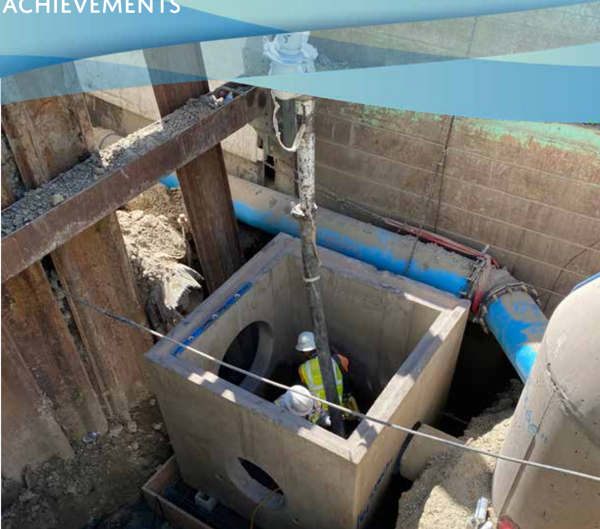
Crew members install a concrete box to house weir gates for the Central San wastewater diversion structure.
