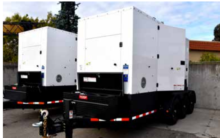
Two of the new portable emergency generators are stationed at the Regional Wastewater Treatment Facility, where they are ready to go online when needed.
