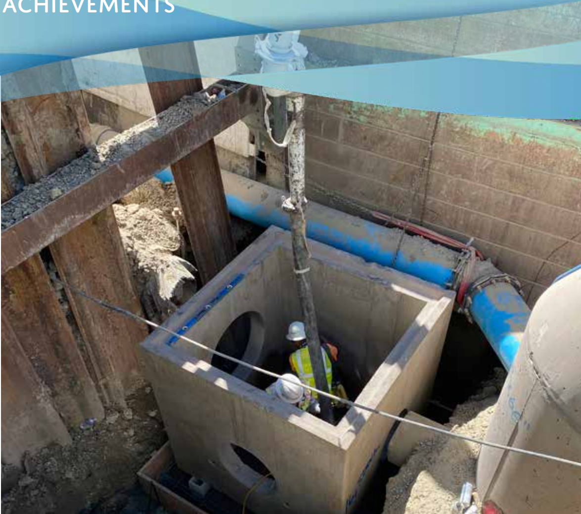
Crew members install a concrete box to house weir gates for the Central San wastewater diversion structure.
