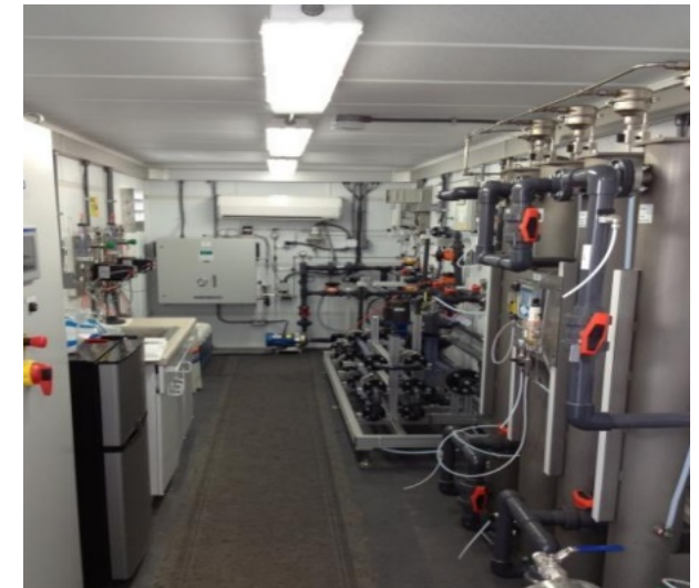
Xylem MiPro containerized O3/BAF 6 and UV AOP system
