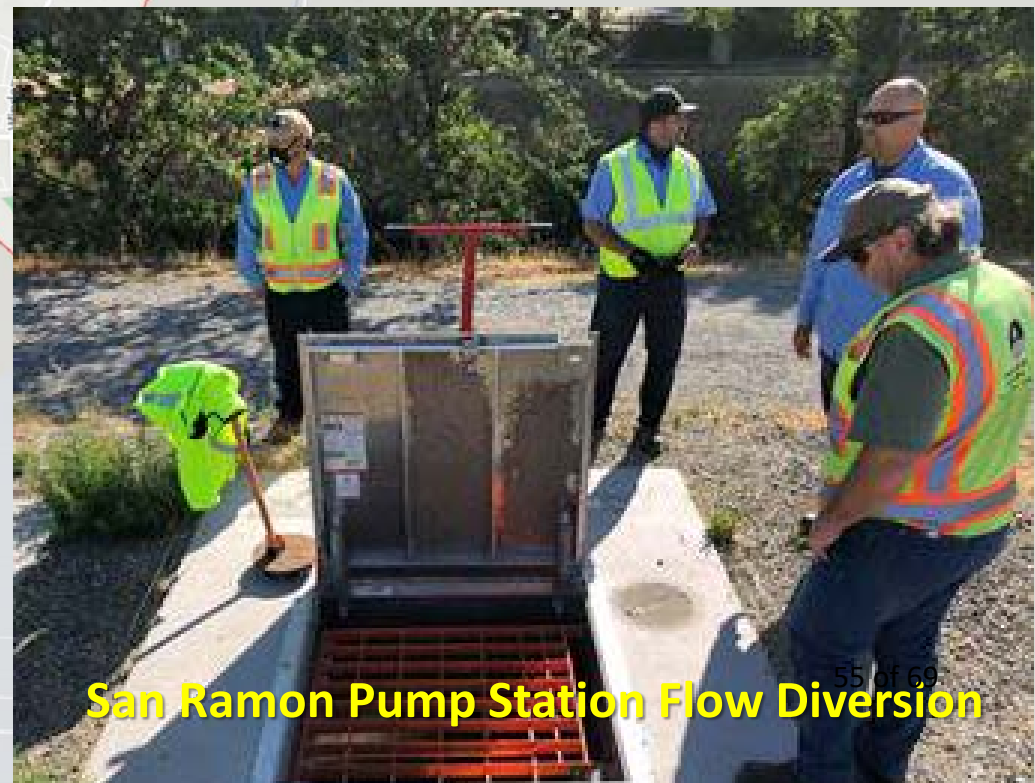
Connection to DSRSD
