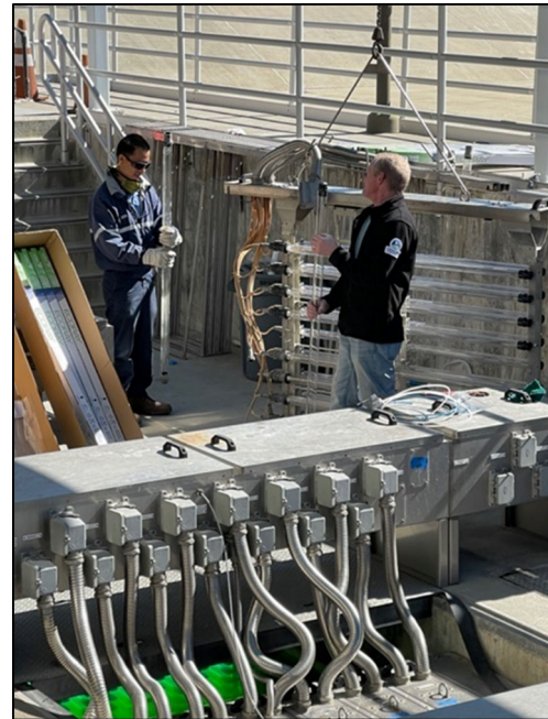
DSRSD staff check the SFUV system to ensure recycled water continues to meet disinfection standards.
