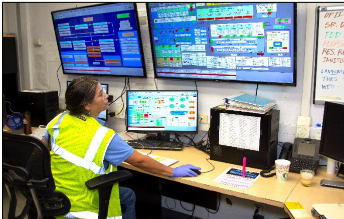
The SCADA control system monitors recycled water production.
