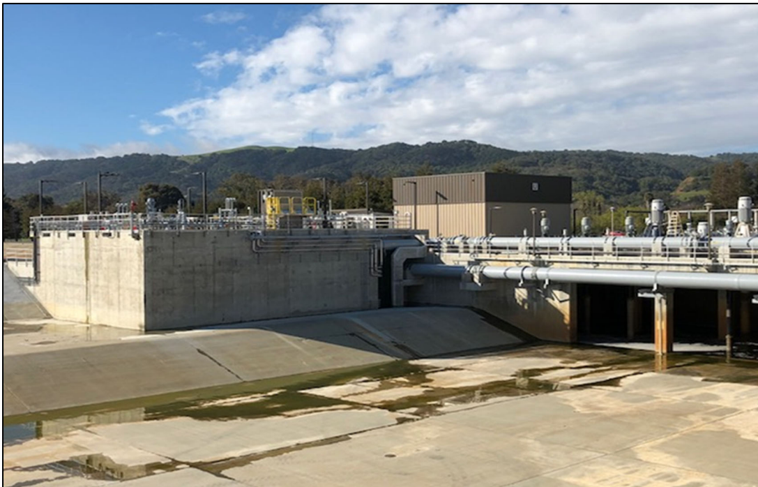
DSRSD basins stand ready to receive and store secondary effluent supply until it begins the ballasted flocculation process.
