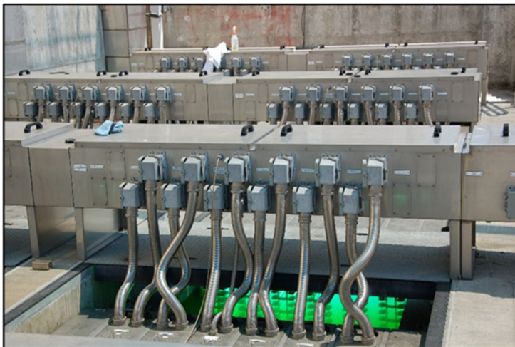
In 2021 DSRSD receive approval to operate the Recycled Water Treatment Facility, including UV disinfection operations, at an increased capacity.
