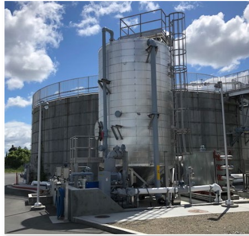
FOG Receiving Station
