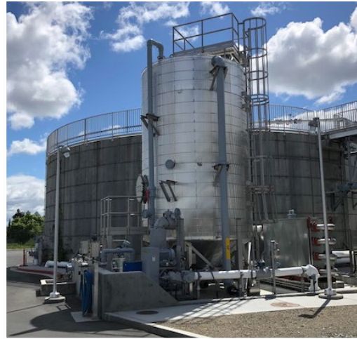
FOG Receiving Station
