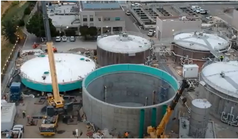
Fourth Anaerobic Digester
