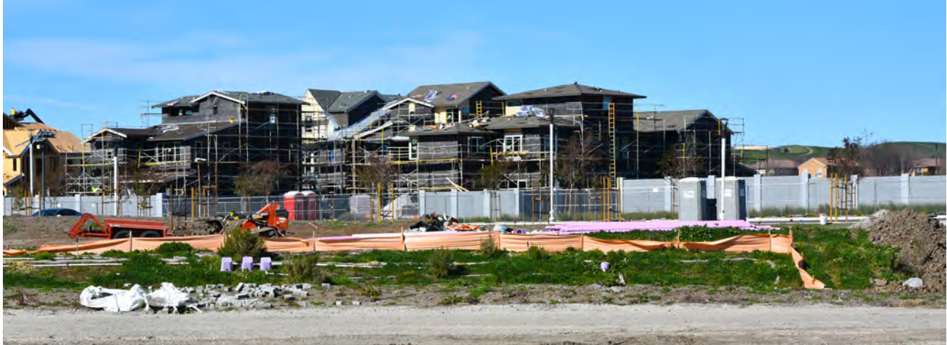
Construction continues on the Boulevard development on the former site of Parks Reserved Forces Training Area in Dublin.
