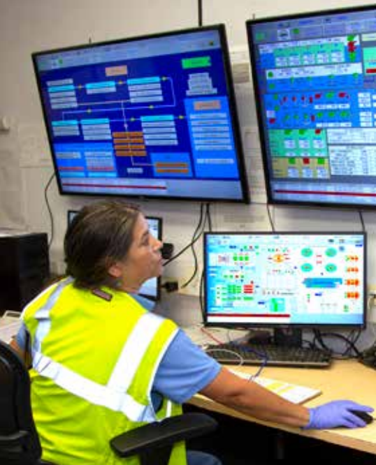
Senior Wastewater Treatment Plant Operator Anna Garcia monitors the Regional Wastewater Treatment Facility's Supervisory Control and Data Acquisition system.
