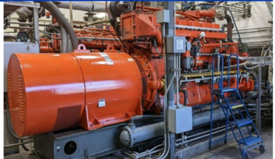
WWTP: Secondary Power Backup
