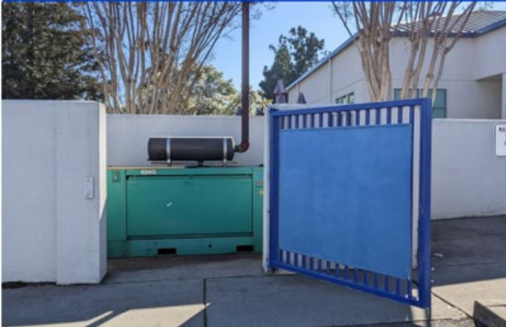
WWTP: Two Standby Generators (Primary)
