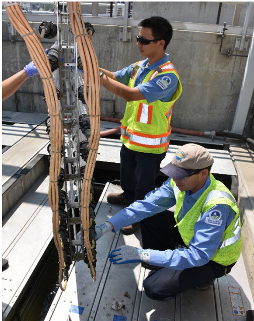
Staff perform maintenance on DERWA's UV system to ensure recycled water continues to meet disinfection standards.
