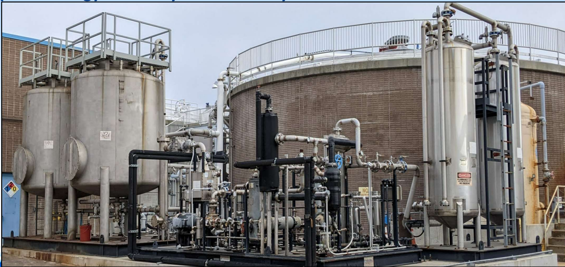
Biogas Treatment System Improvements ($3.0M)
