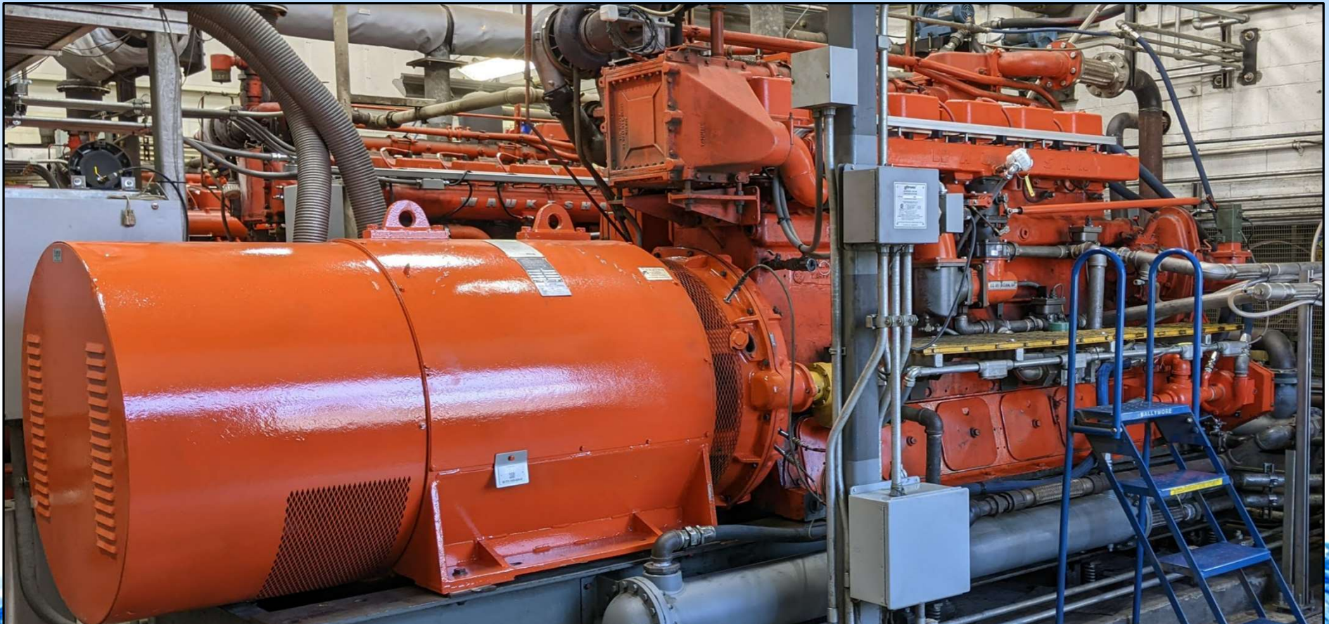
Cogeneration Engine Replacement (FYE 28-31: $33.5M)
