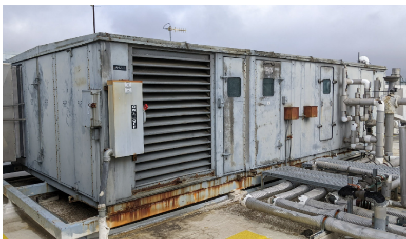
Figure 2 Air Handling Unit
