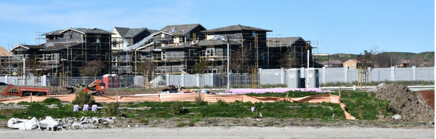
Construction continues on the Boulevard development on the former site of Parks Reserved Forces Training Area in Dublin.
