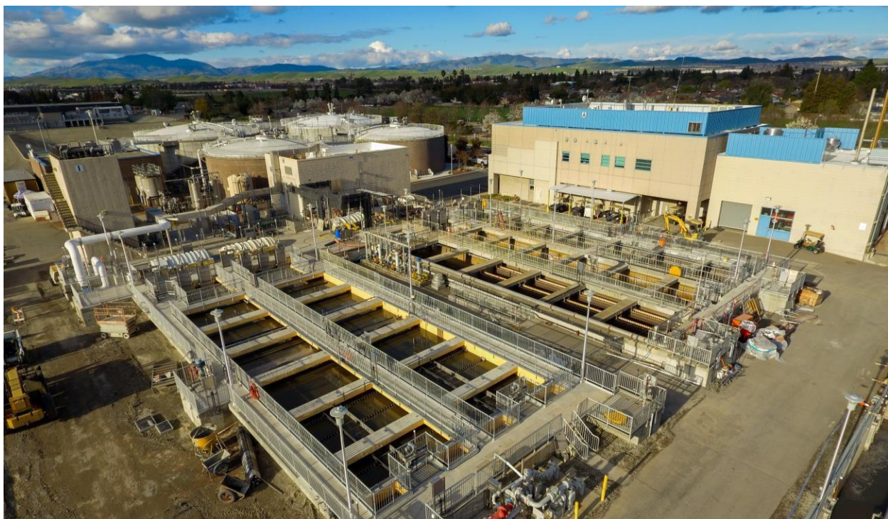
DSRSD's Regional Wastewater Treatment Facility is located in Pleasanton and treats domestic, commercial, and industrial wastewater.
