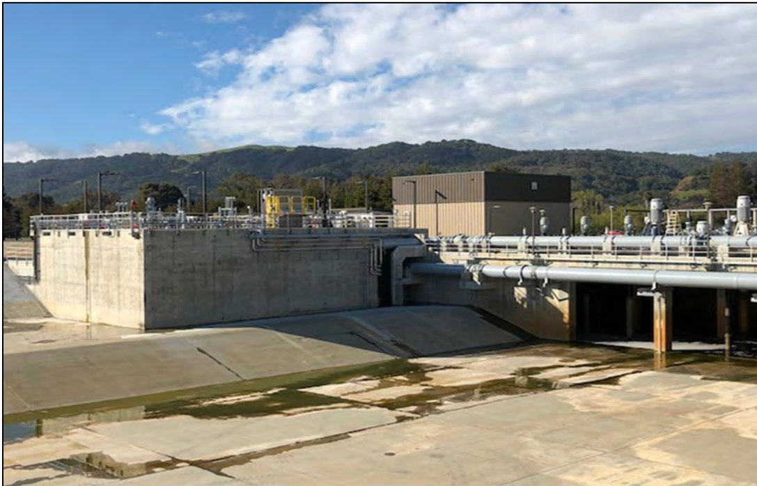
DSRSD basins stand ready to receive and store secondary effluent supply until it begins the ballasted flocculation process.
