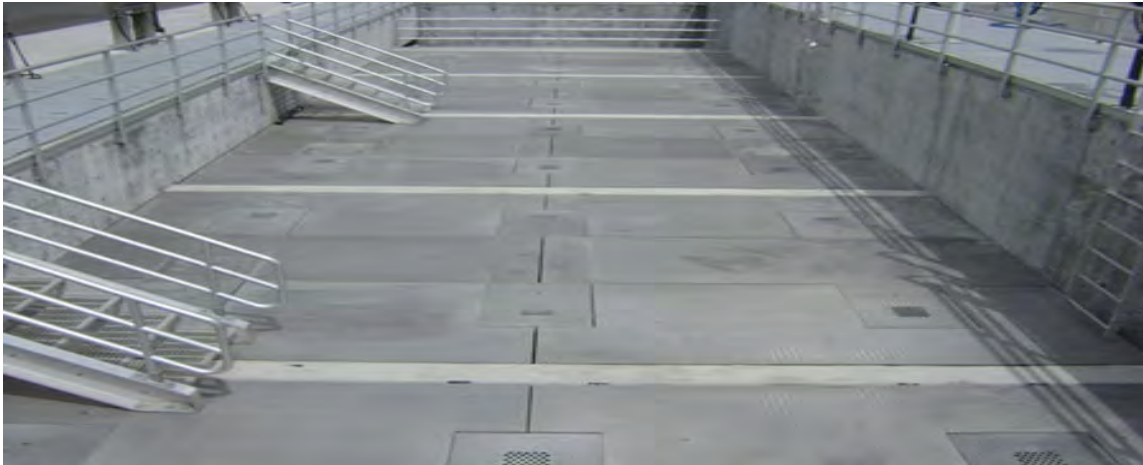
Access plates hide six sand filters where flocculated water flows upward through 80 inches of continuously backwashed sand.
