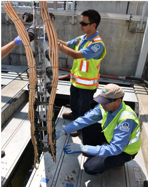
Staff perform maintenance on DERWA's UV system to ensure recycled water continues to meet disinfection standards.
